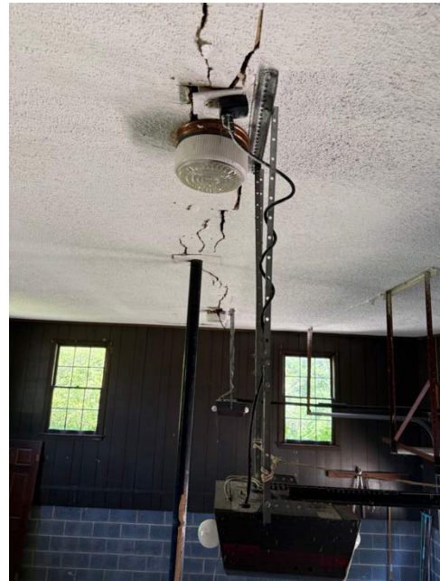
Resulting crack in ceiling
